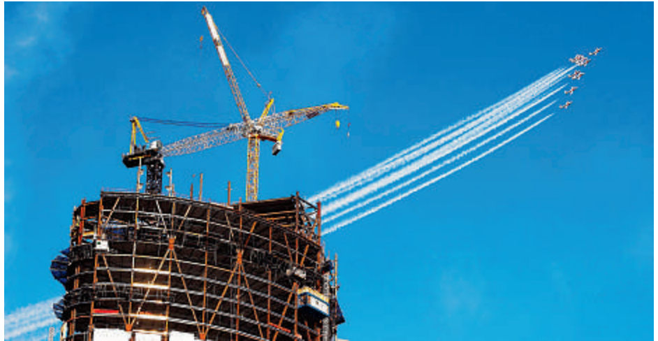
Western Canadian landmark: The Bow office and retail project, seen as the Canadian Forces Snowbirds fly past before the 2010 Calgary Stampede parade, will be Canada's second-tallest.
